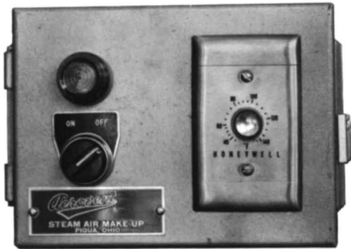
Remote Operating Station with outlet temperature control (OTC) selector, on-off switch, and indicator lamp at floor level
