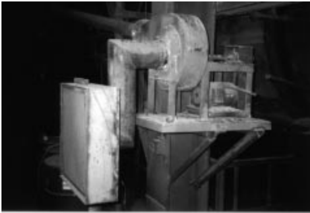
Figure 7. Poorly-designed duct configuration
